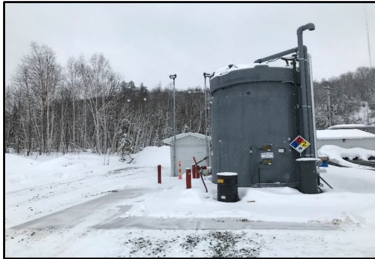
New sulfuric acid tank installed near former acid tote storage building, 2020.
