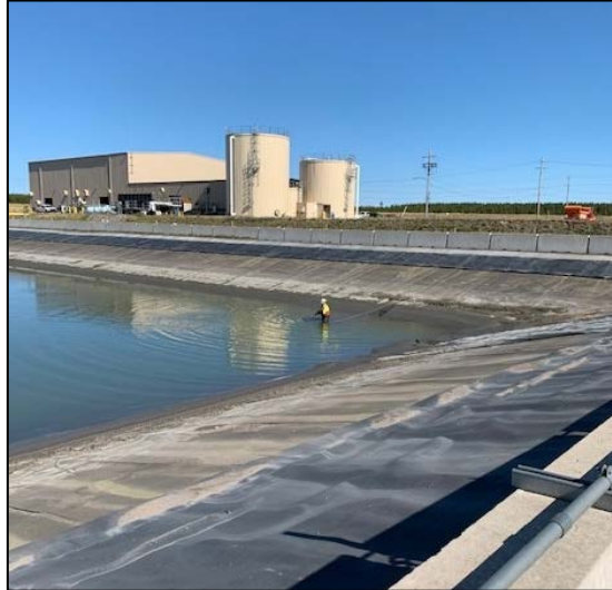
Follow Up Inspection to Leak Location Survey in CWB #2, September 2021
