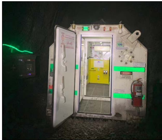
Underground Refuge Chamber
