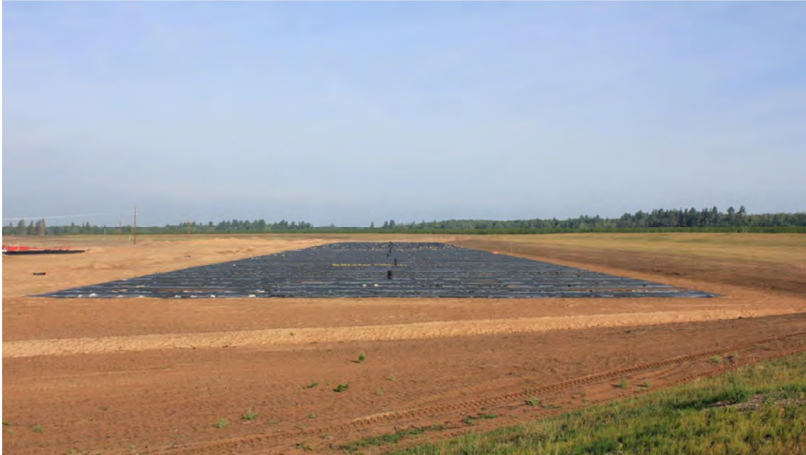
Treated Water Infiltration System (TWIS), September 2011
