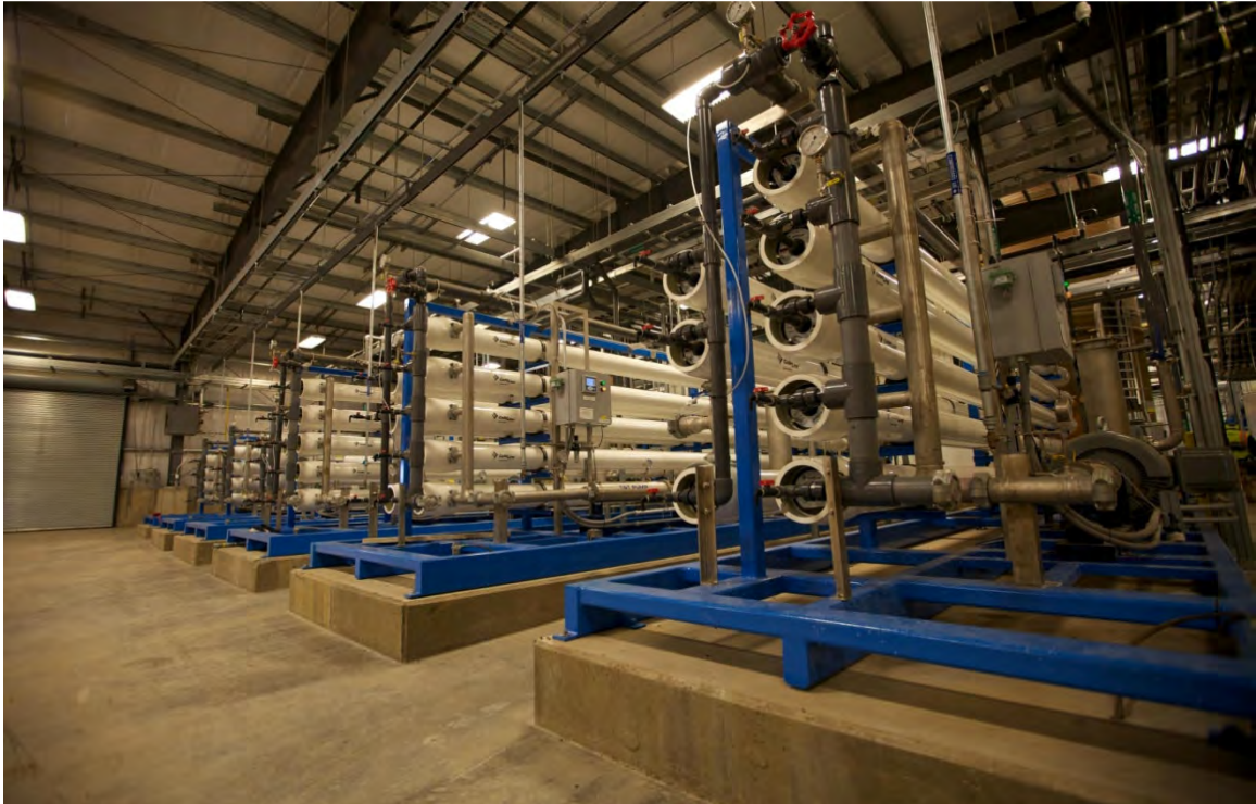
Reverse Osmosis Units in WTP, 2011
